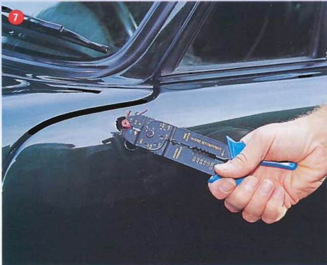
7 Strip back the black sheath and then crimp a female connector to the end of each of the five wires coming from the door. Check that each connector is firmly attached; they can work loose
